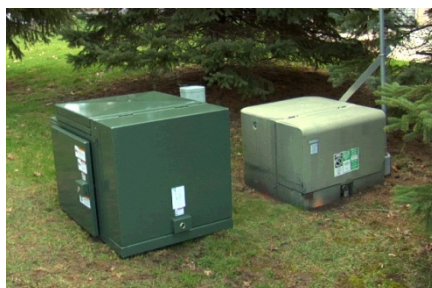
Community Energy Storage
